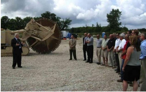
Pat Riordan, president and CEO of Cellcom, addresses a group of Door County business and government leaders August 4th about the company's plans to run a fiber-optic network from Green Bay to Sturgeon Bay. He is standing in front of a massive Tsmec machine that can cut a trench through Door County's rocky terrain.
